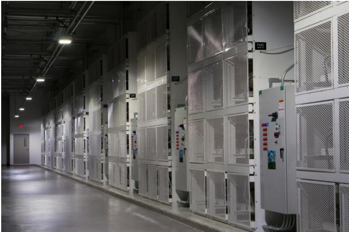
Slika 2: Ventilatori u Facebookovu podatkovnom centru prema izvoru: https://techcrunch.com/gallery/a-look-inside-facebooks-data-center/slide/20/ , preuzeto 31.8.2020.
